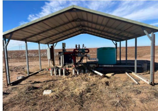
W Drip Station
